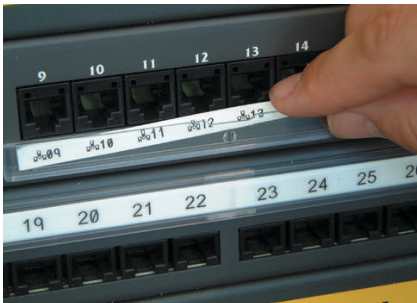
Punch block & patch panel labels
